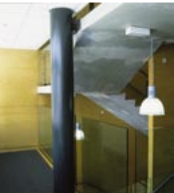
Above: All non-structural steelwork in the complex was finished in Resene's Lusta-Glo semi-gloss enamel in Zeus.
