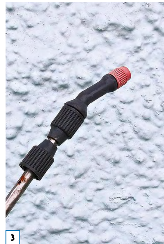
3 Spray the stucco with the Resene Moss & Mould Killer solution and leave for 48 hours.
