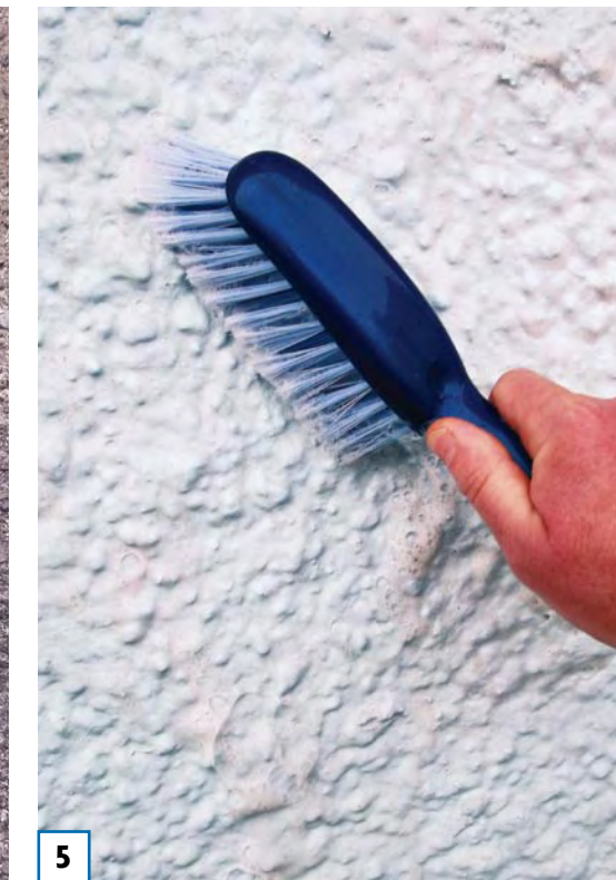
5 Using the stiff-bristled brush, scrub the stucco vigorously, ensuring the Resene Paint Prep and Housewash solution is worked into the surface of the wall. Once thoroughly washed, rinse clean with plenty of cold water. Allow to dry.
