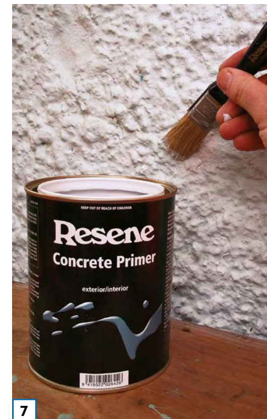
7 Spot prime the filler and any patches of bare concrete with Resene Concrete Primer. Allow two hours to dry.
