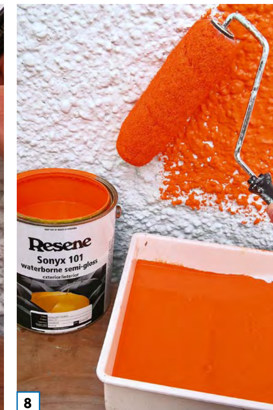
8 Apply two coats of Resene Sorbus to the wall, allowing two hours for each coat to dry. ■
