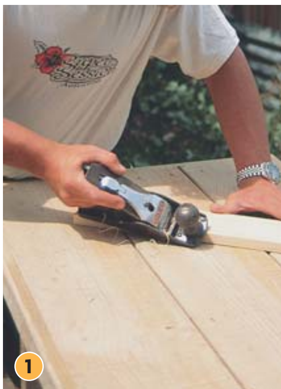
1 Cut the base legs to the dimensions given. Plane the seat slats on the top edges.
